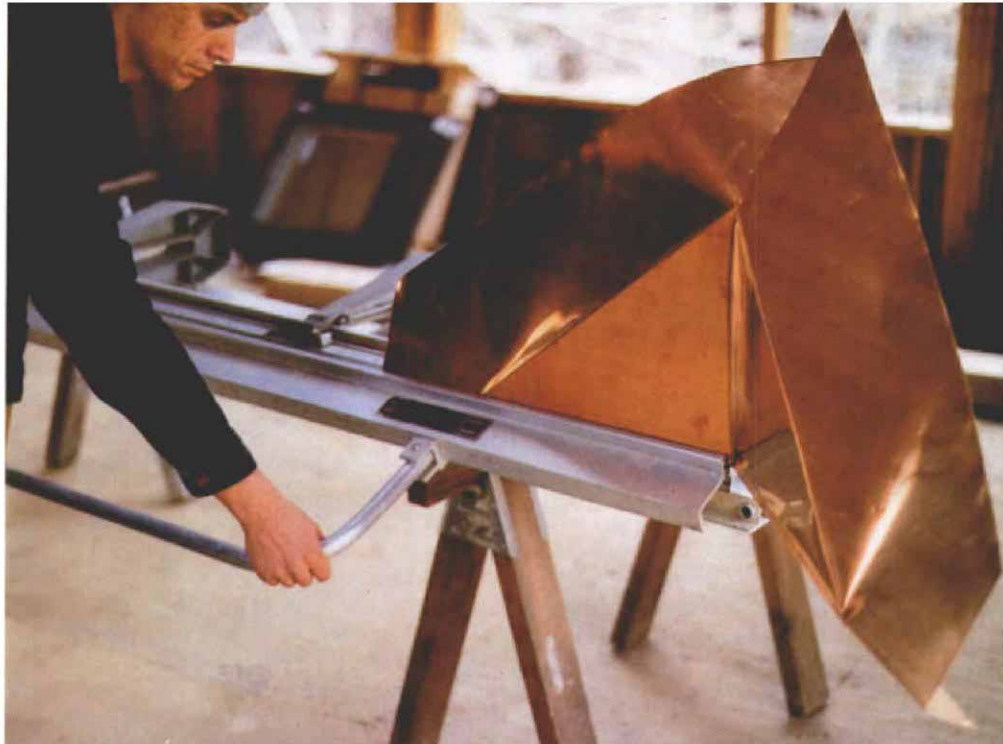
Most of the folds were made on the metal brake shown above. Eventually the configuration of bends prevented the roof sheet from slipping into the brake, so the final folds were handmade.
