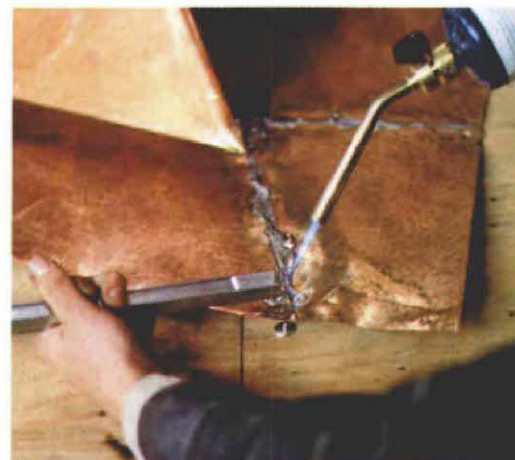
McBride solders the flashing in his shop, instead of on the roof. This way he can position the flashing so that the seams are level when he solders them, which keeps the molten solder from running out of the joint.
